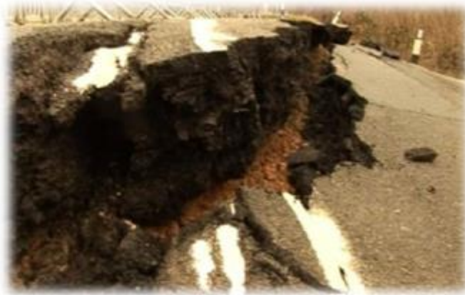
Oxford Road in Bagley Wood collapsed after the heavy rain in November 2012 saturated the ground. The road reopened a year later. Repairs cost £1 million.
